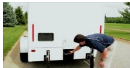
Accessible 4" Clean Out Port.
