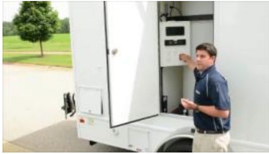
Battery Disconnect in unit
