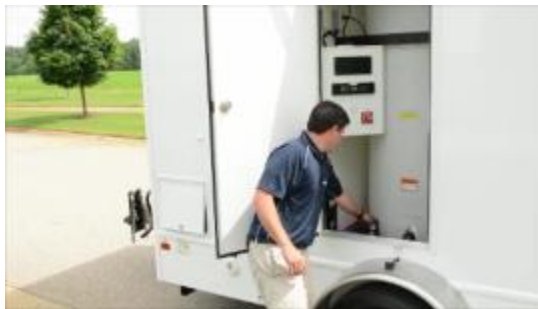
Pressure Gauge in Unit.
