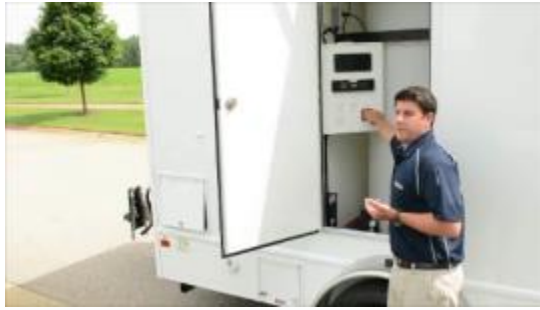
Battery Disconnect in unit
