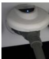
Check Blue Light on Trailer
