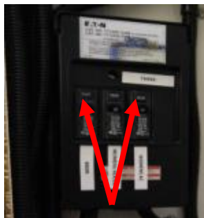
Men's AC Breaker
