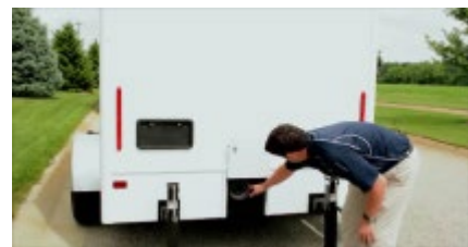
Accessible 4" Clean Out Port.
