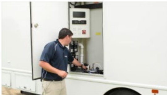
Pressure Gauge in Unit.
