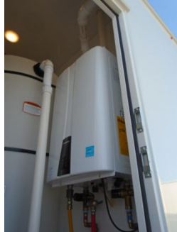
Back Water Heater
