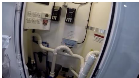
Service Area Outlet
