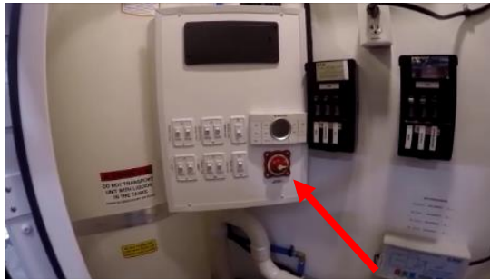
Battery Disconnect in unit
