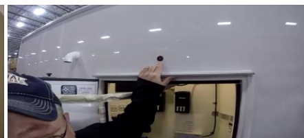
Indicator Light (60 Flushes)
