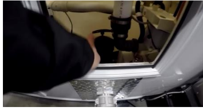
Accessible 4" Clean Out Port.
